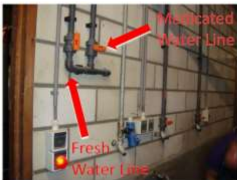
Two water lines were available with one dedicated to delivering medication. Valves within the housing allowed control of medication to the individual pen level.
